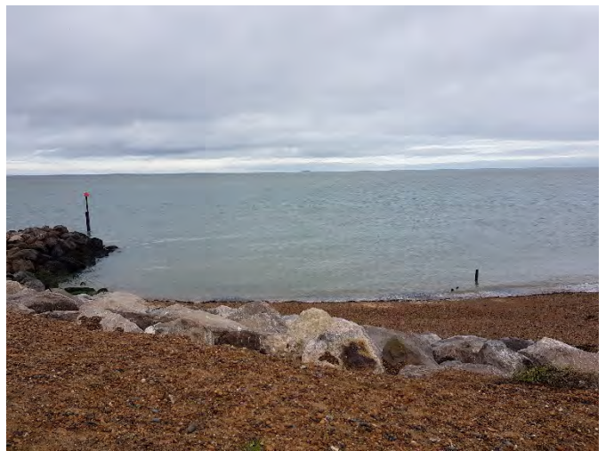
Coastal defences and submerged groyne looking out to sea
