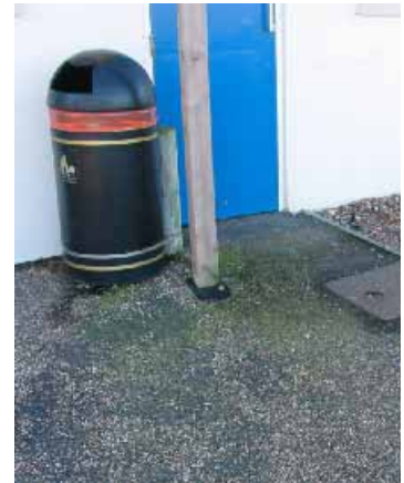
poorly located and unattractive
