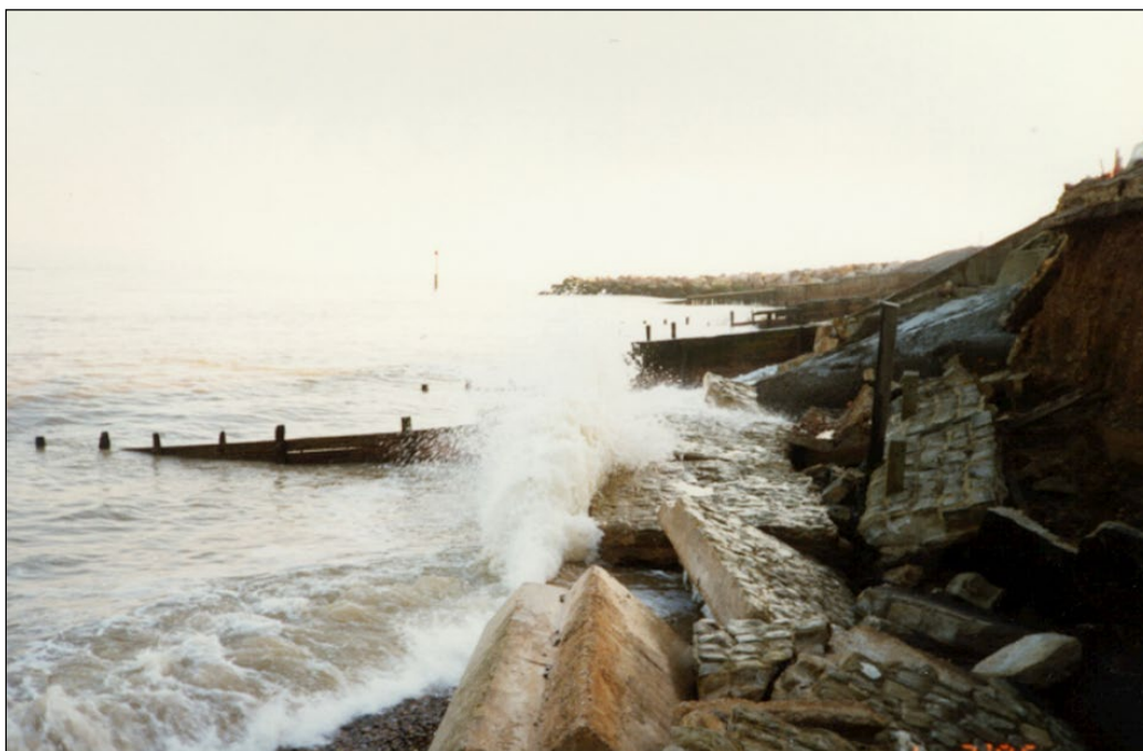
Figure 4.4 - Failed Seawall at Reculver caused by the 1996 Storm.
