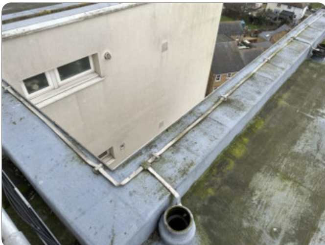
Fire Hazards (Photo 3)
