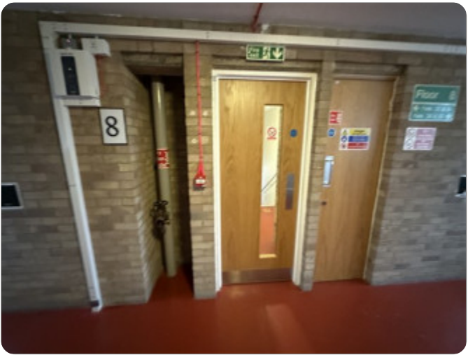
Fire Protection (Photo 11)
