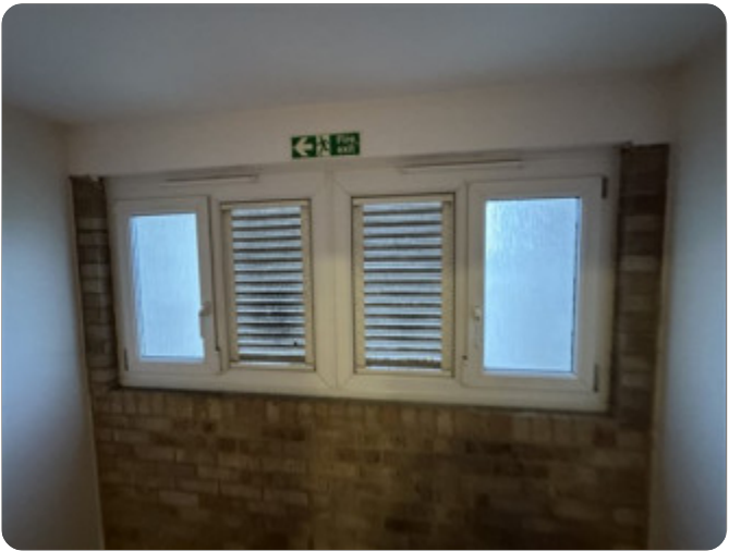
Fire Protection (Photo 13)
