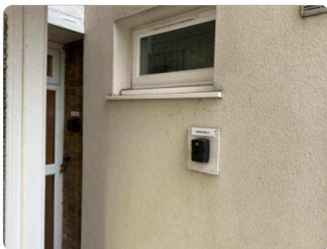
Fire Protection (Photo 5)
