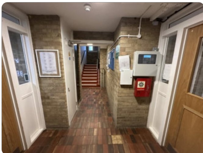
Fire Protection (Photo 18)
