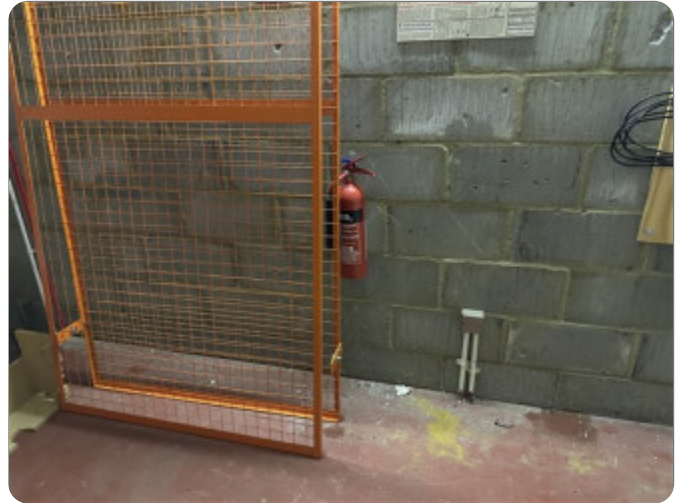
Fire Protection (Photo 21)
