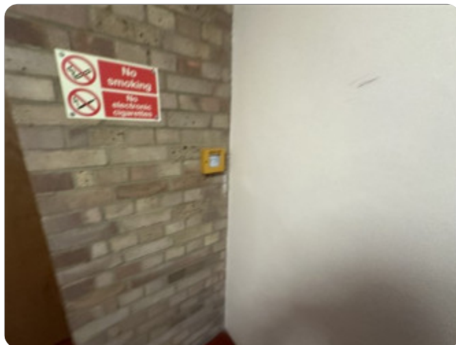
Fire Protection (Photo 15)
