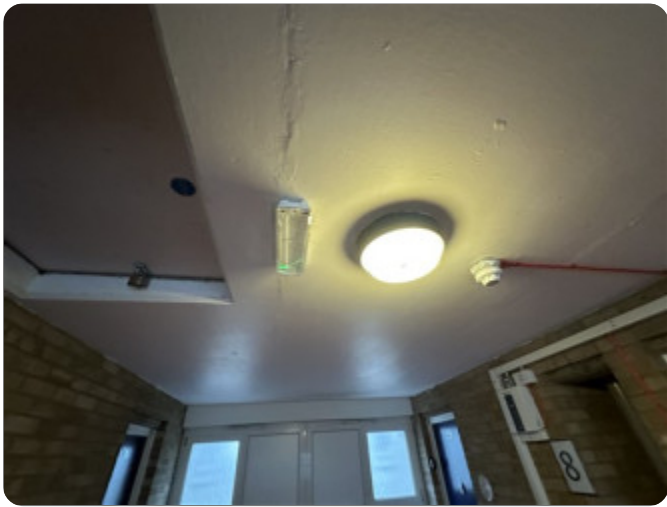
Fire Protection (Photo 10)
