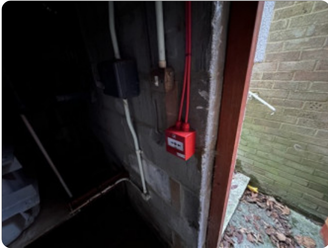
Fire Protection (Photo 20)
