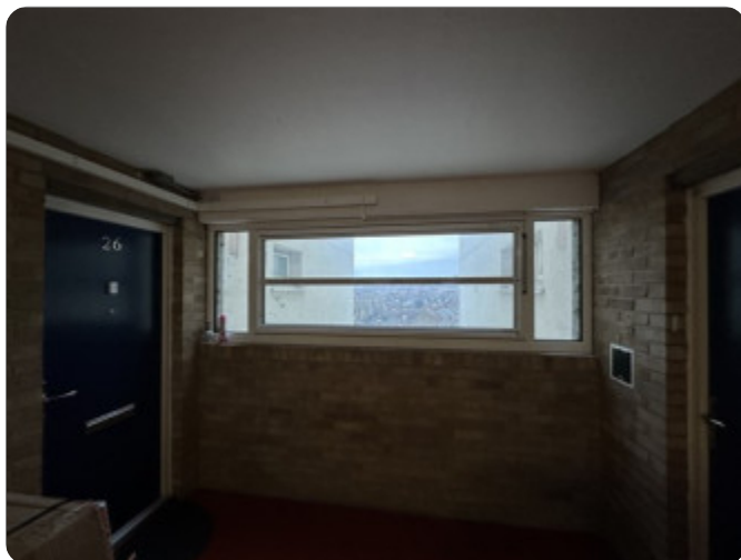
Fire Protection (Photo 14)
