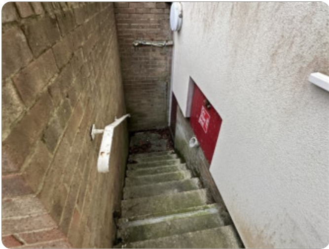
Fire Protection (Photo 12)
