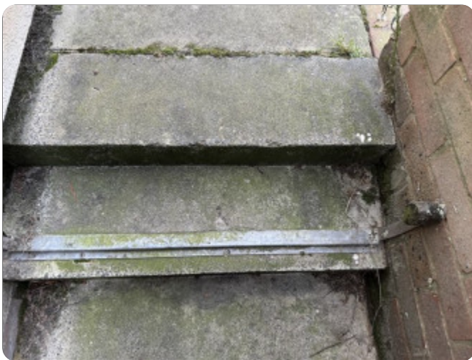
Fire Hazards (Photo 1)
