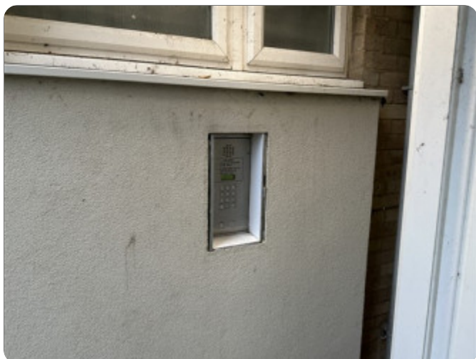
Fire Protection (Photo 6)
