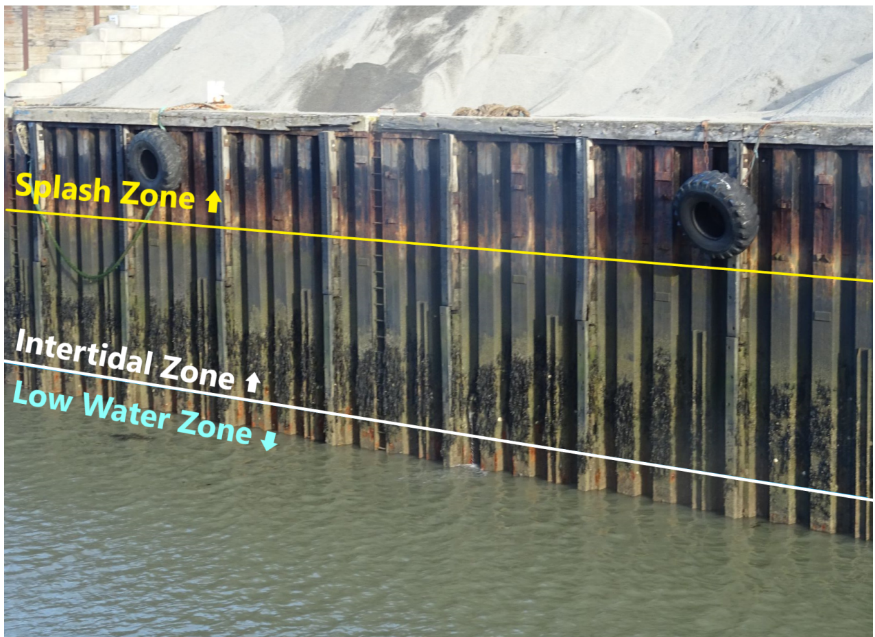
Steel sheet pile corrosion zones
