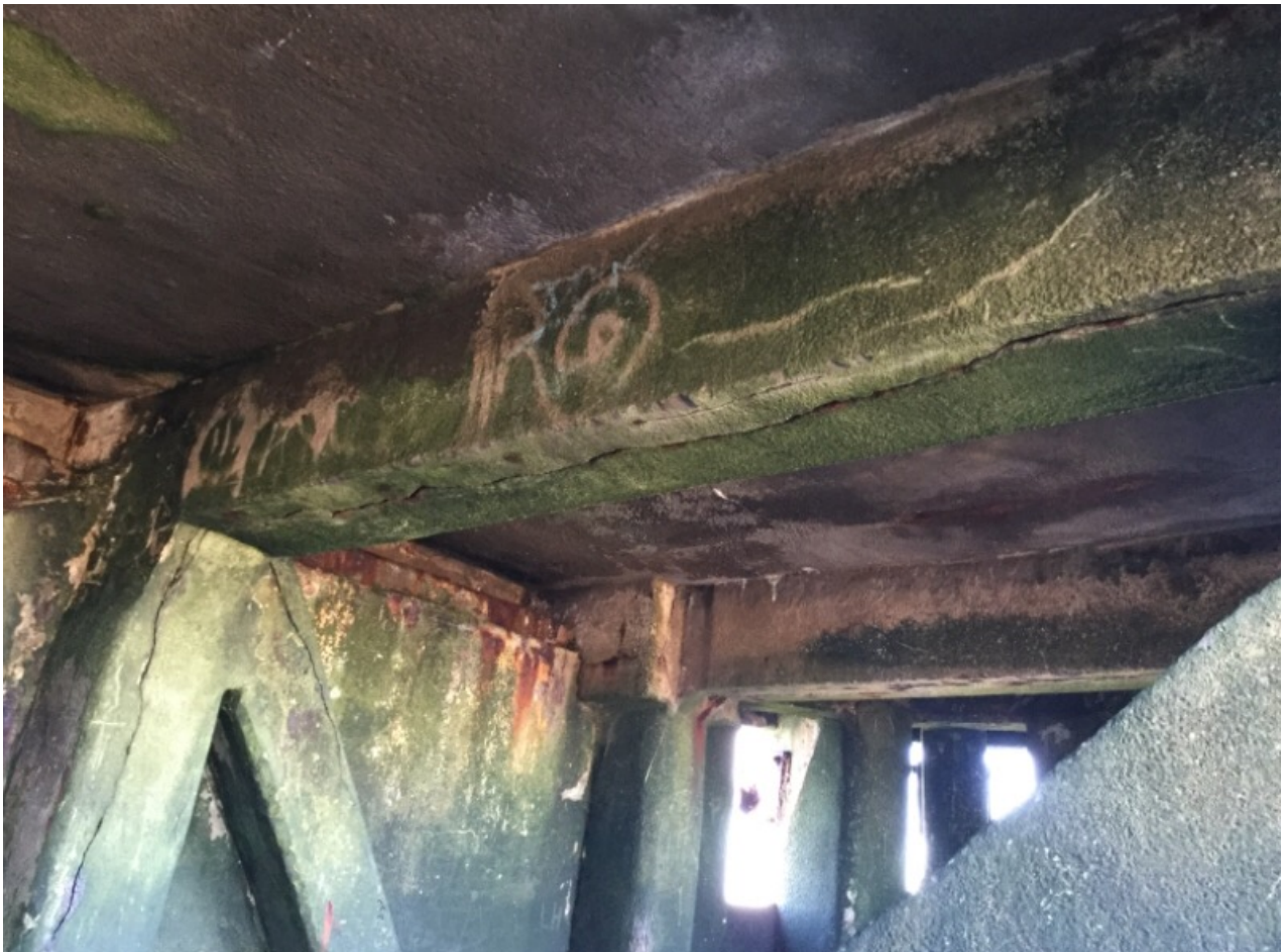
Cracking to the support beam underneath the East Quay Pier Head
